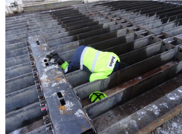
Place where accident happened notice slippery stopper.
