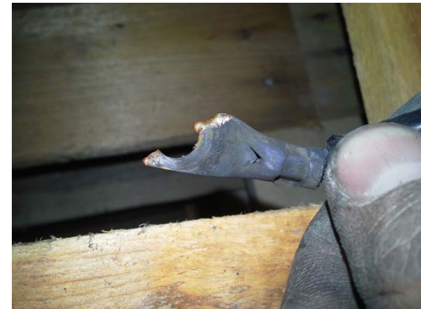
The connector of the plus pole on the frame under the fastening screw of the last (no. 4) battery melted as a result of the short-circuit.
