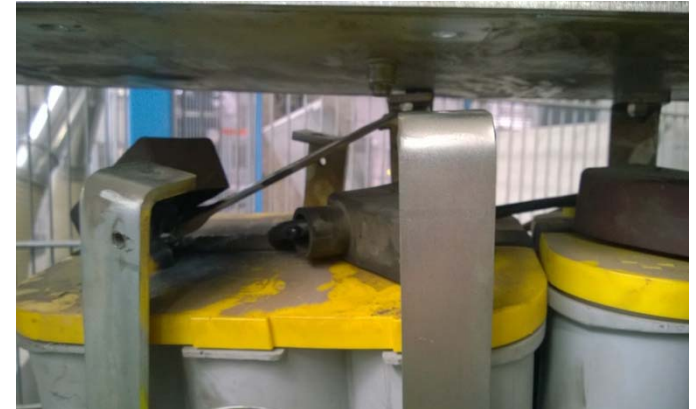
The spanner was caught between the plus pole and the nut causing a short-circuit and arcing.
