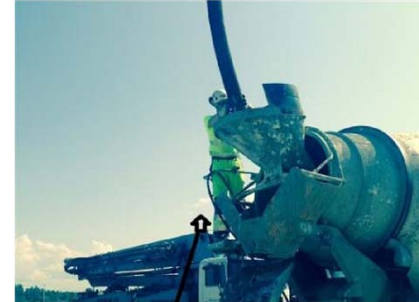
The driver fell down from the work platform on his right side. The height of the platform is ca 2.5 metres.
