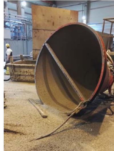
Concrete hopper fallen on the floor.
