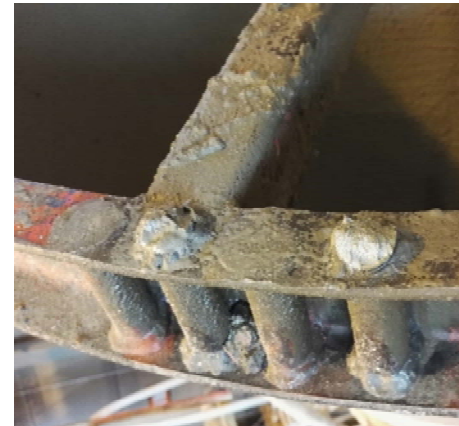
Broken lifting lug on the concrete hopper.
