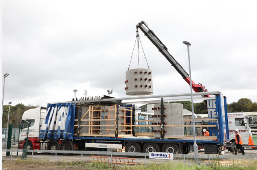
Lifting of the drawpits out of the truck which came from Finland
